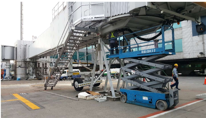
An ABB is being installed on site.
